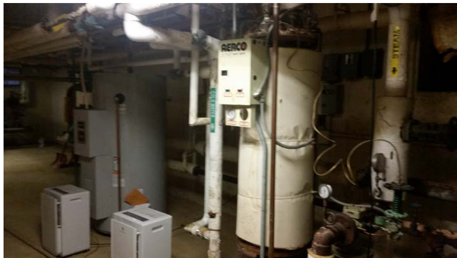
Typical Mechanical Room (Building 18)
