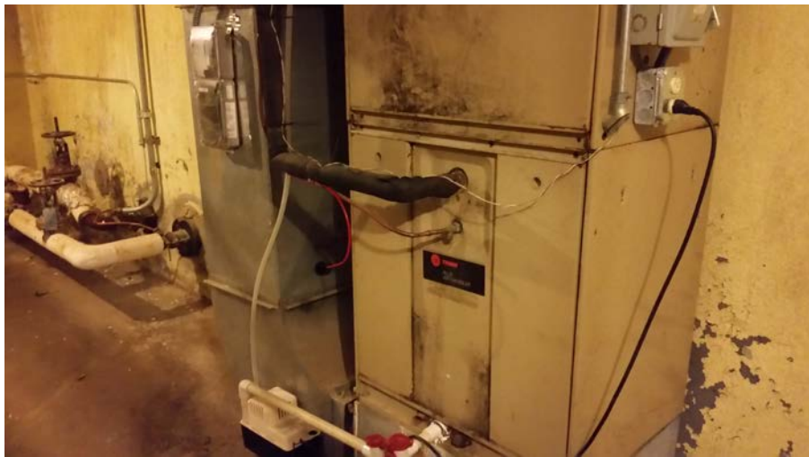
Typical Mechanical Room (Building 18)
