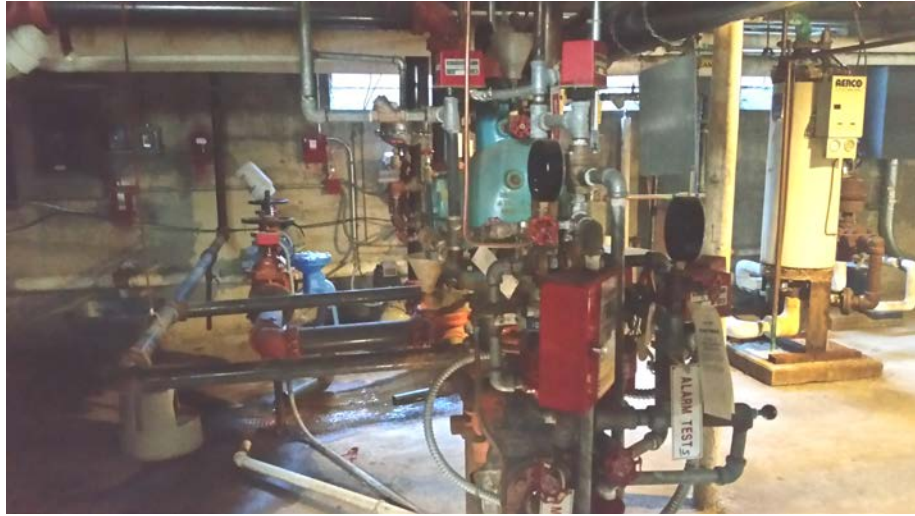
Figure 3: Mechanical Equipment Room (Building 18)
