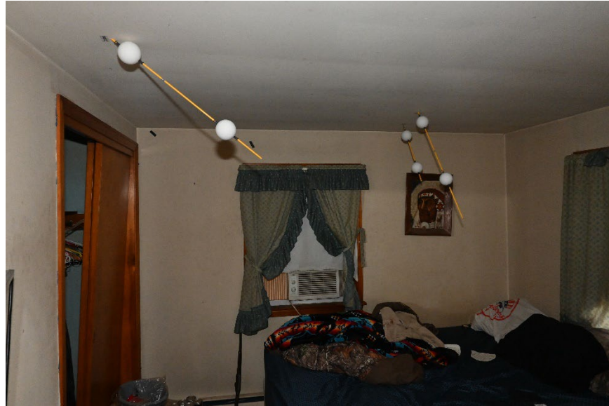
[Trajectory rods in bullet defects in ceiling]
