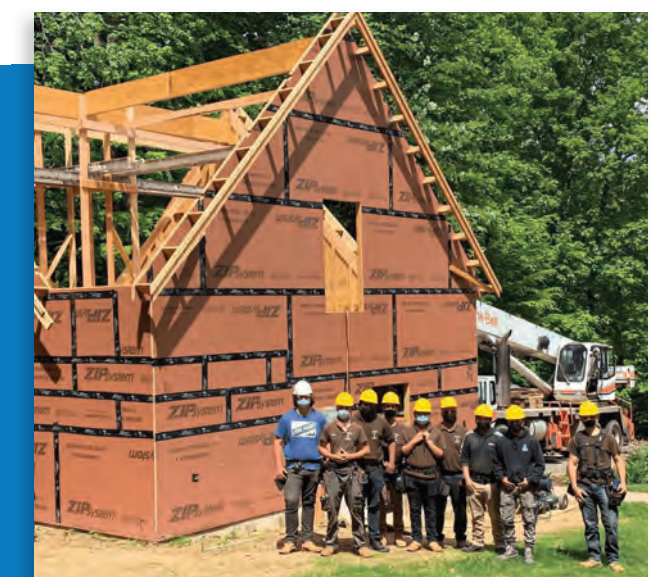
Abbott Tech Carpentry Juniors construct a three-car garage with a full loft.
