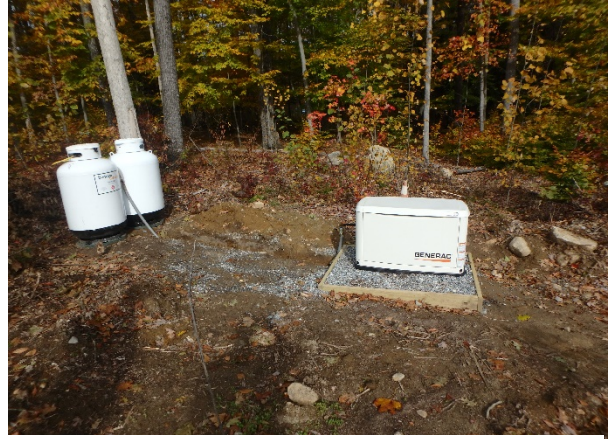
Garden Lane Apartments – Emergency Generator & Propane Fuel Tanks
