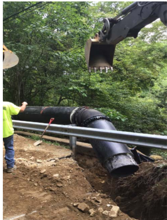
Norwich Public Utilities- Stony Brook Transmission Main Rehab Installation of Insulated Water Main Across Culvert Crossing
