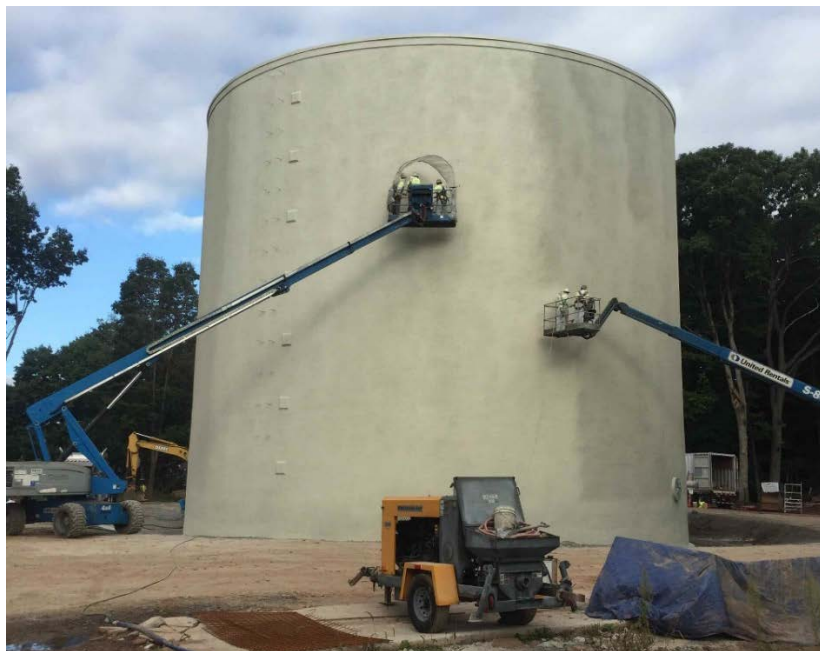
Southington - New Mill St. Tank
