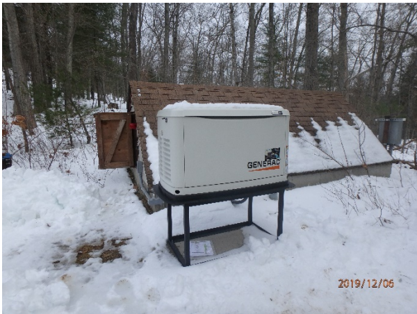
Willington Ridge – Emergency Generator
