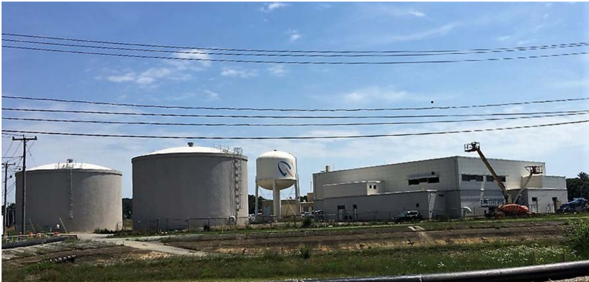
Groton Utilities-Water Treatment Plant Upgrade Project Panoramic View of New DAF and Filters Building and New Storage Tanks
