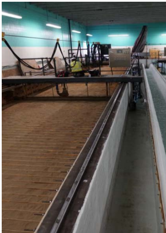
Norwich Public Utilities-Deep River Filters Rehab New Filter Media at Filter Unit #2
