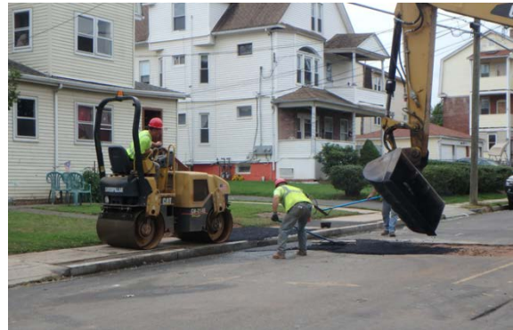
MDC – Bond St. Water Main Replacement Paving after Water Service Line Replacement
