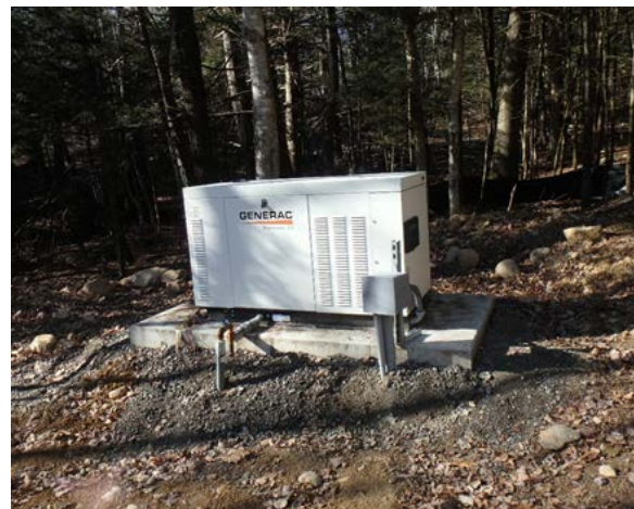
Ashford Hills – Emergency Generator
