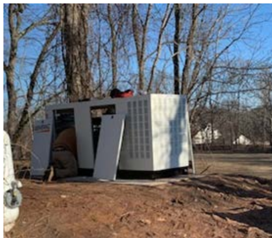
Yeshiva Gedolah of Waterbury –Emergency Generator
