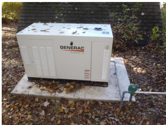
Brookwoods II –Emergency Generator
