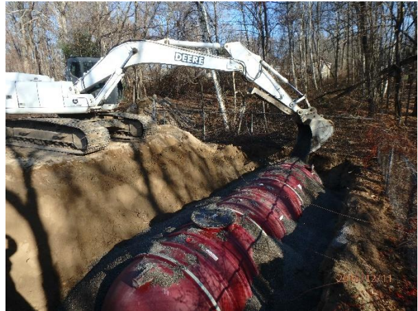
Woodland Summit – New water storage tank
