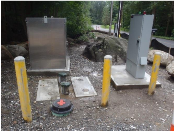
Bethel – New Booster Pump Station
