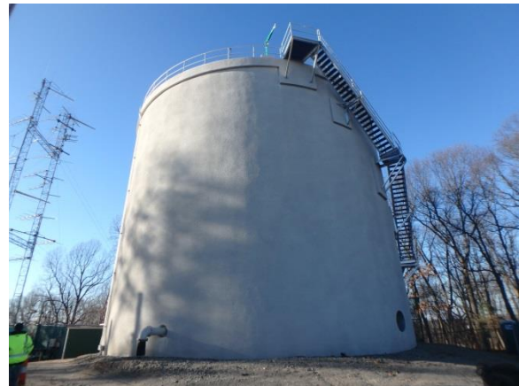
RWA – Completed Burwell Hill Tank
