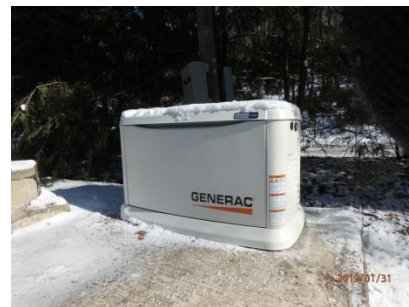
Candlewood Springs – Finished Generator
