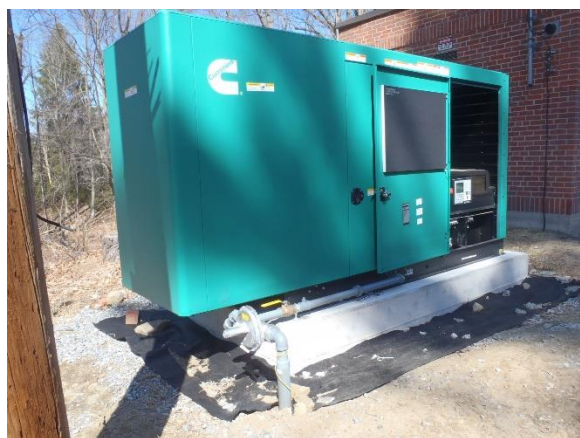
Waterbury – Pump Station Generator
