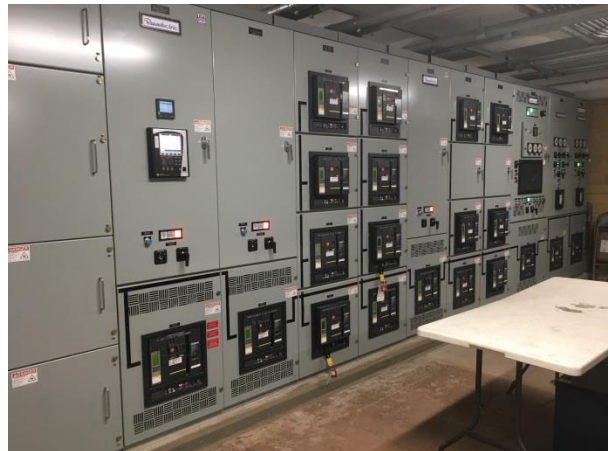
Groton Upgrade – Electrical Control Room
