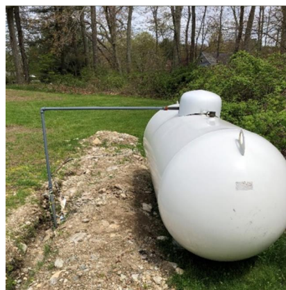
Arnio Drive – Propane Gas Tank
