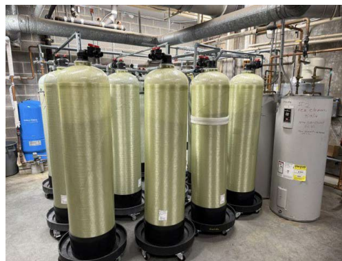
KILLINGWORTH ELEMENTARY SCHOOL - POINT-OF-ENTRY TREATMENT - PFAS & OCCT, GAC FILTERS, KILLINGWORTH
