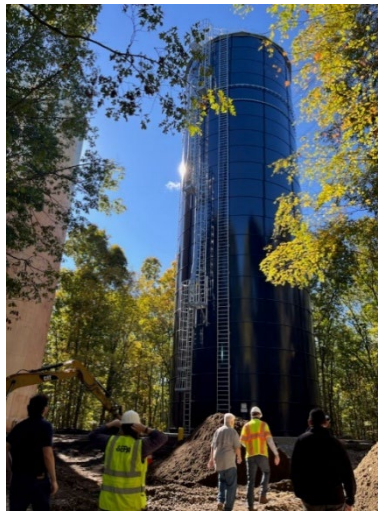
MONTVILLE WATER SUPPLY - 531,200-GALLON TANK, MONTVILLE
