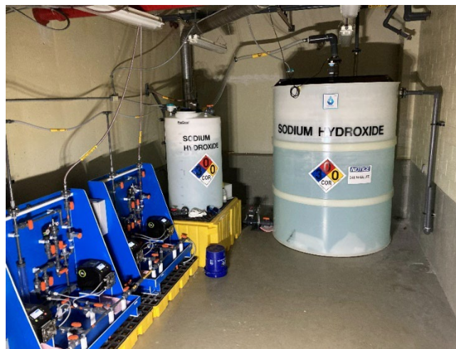
REGIONAL WATER AUTHORITY, LAKE WHITNEY WTP TEMP CAUSTIC, HAMDEN
