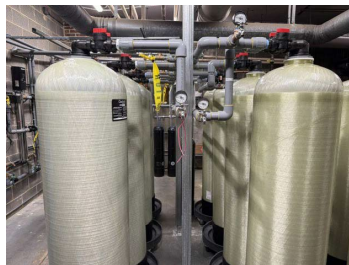
KILLINGWORTH ELEMENTARY SCHOOL - POINT-OF-ENTRY TREATMENT - PFAS & OCCT, GAC FILTERS, KILLINGWORTH
