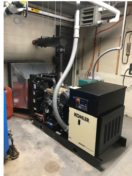
Bethel –Emergency Generators – Briar Cliff Pump Station (above) & Eureka Water Treatment Plant (below)
