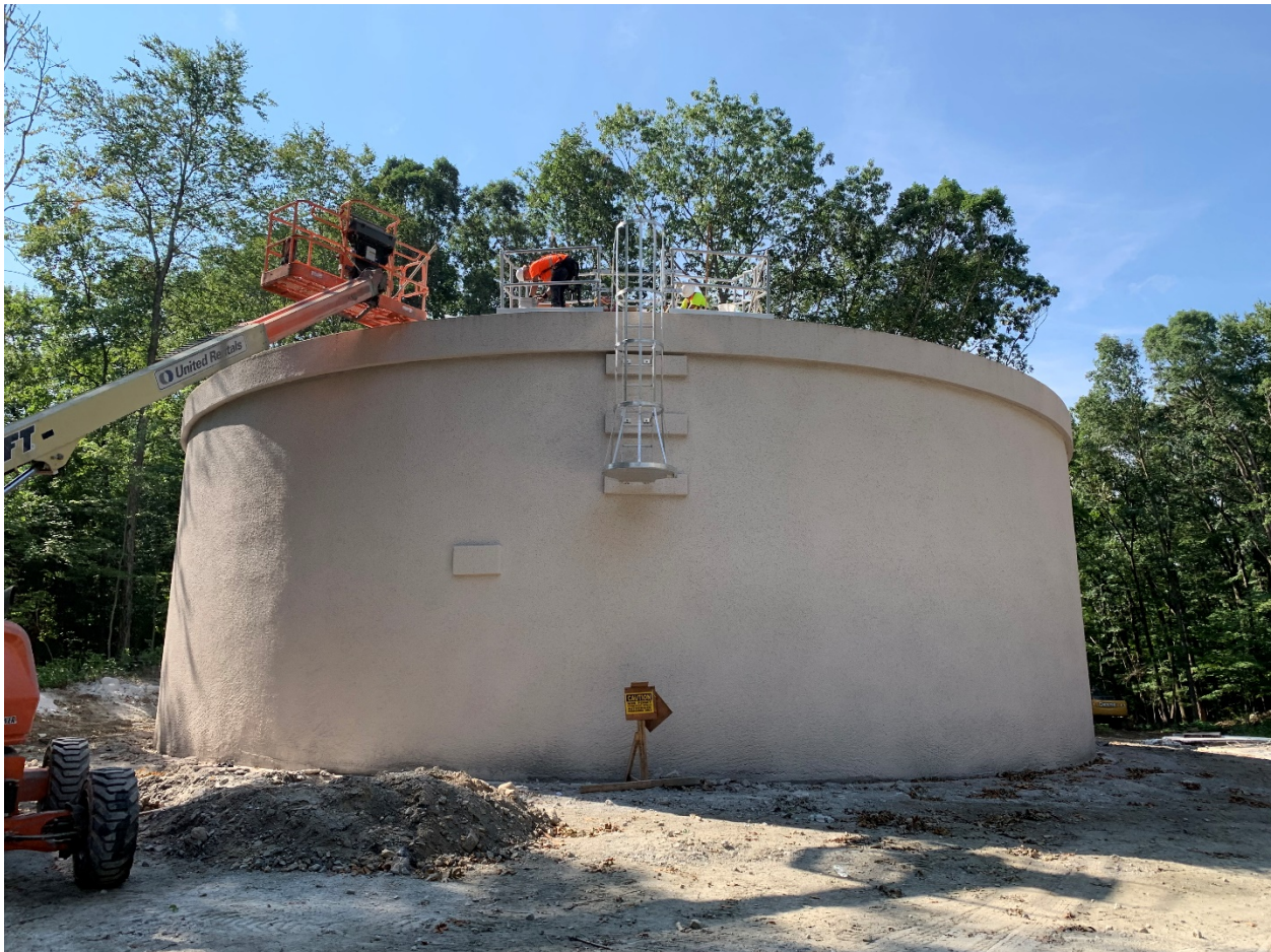
Bethel - New Chestnut Ridge Water Storage Tank
