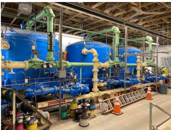
East Lyme – Filtration Treatment Vessels
