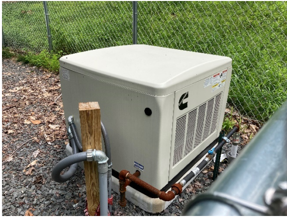
Old Indian Trail – Emergency Generator
