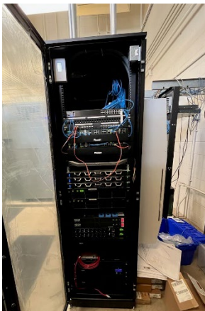
SCADA UPGRADE, BRISTOL CT
