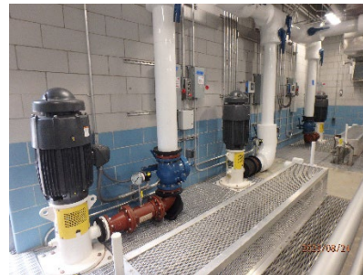
SCCRWA DAF FILTER PUMPS
