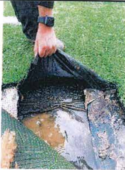
Ponding over e-layer
