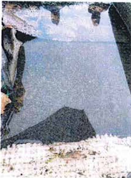
Ponding over e-layer
