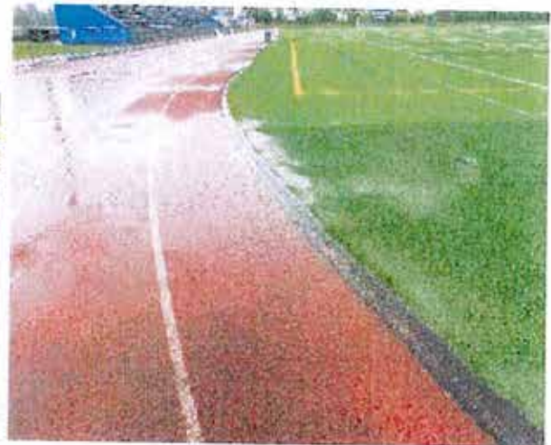
Ponding on Track
