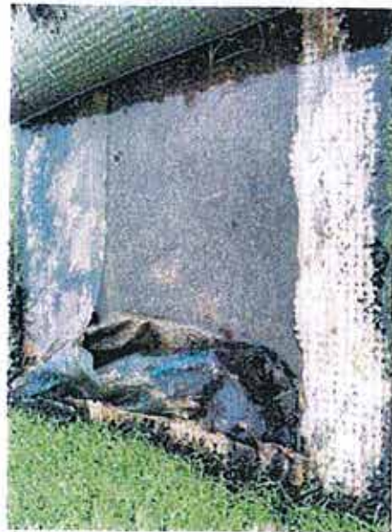
Ponding over e-layer
