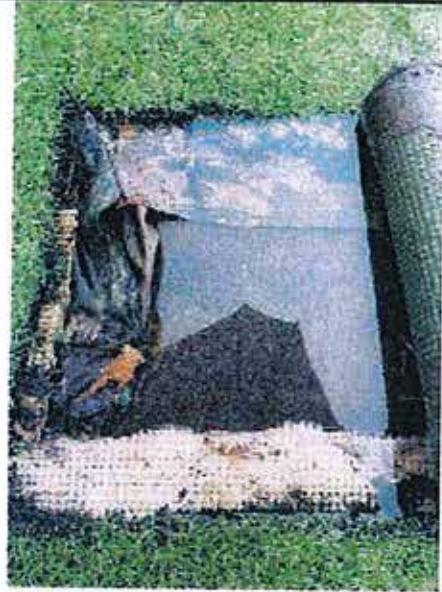
Ponding over e-layer
