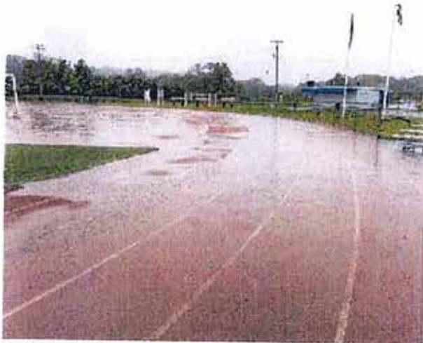
Ponding on Track
