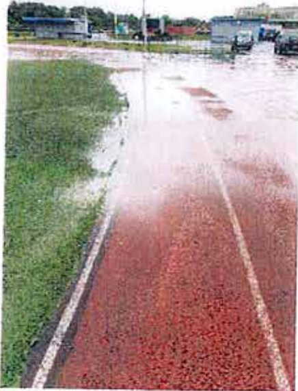
Ponding on Track
