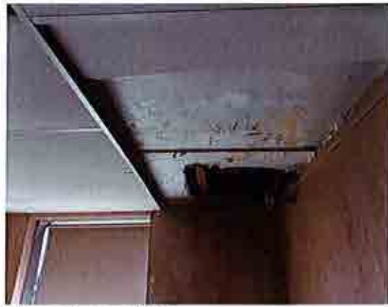
Ceiling damage from roof leak
