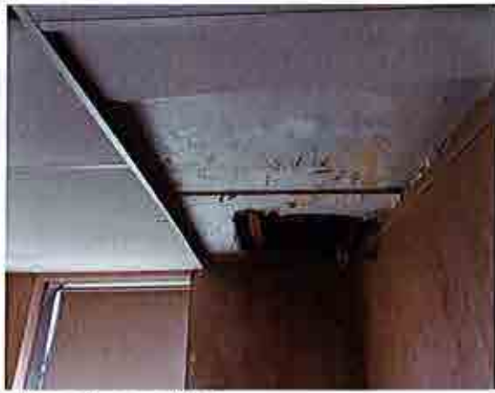
Ceiling damage from roof leak
