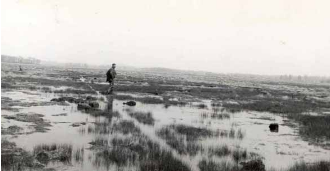
Figure 1. Restoring marsh hydrology by plugging of old mosquito ditches in Connecticut (ca.1938).
