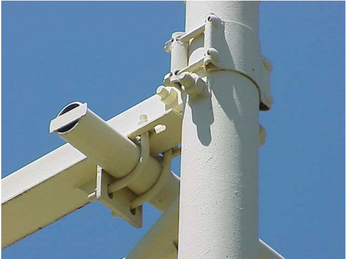
Figure 7 Detail Showing Typical U-Bolt Used in Connection Between Horizontal Truss and Vertical Supporting Truss
