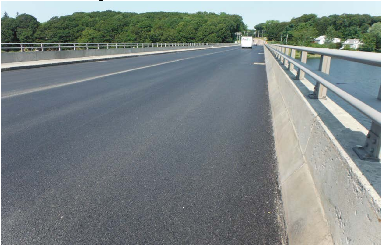
Figure 5. General Condition of HFTL Mix
