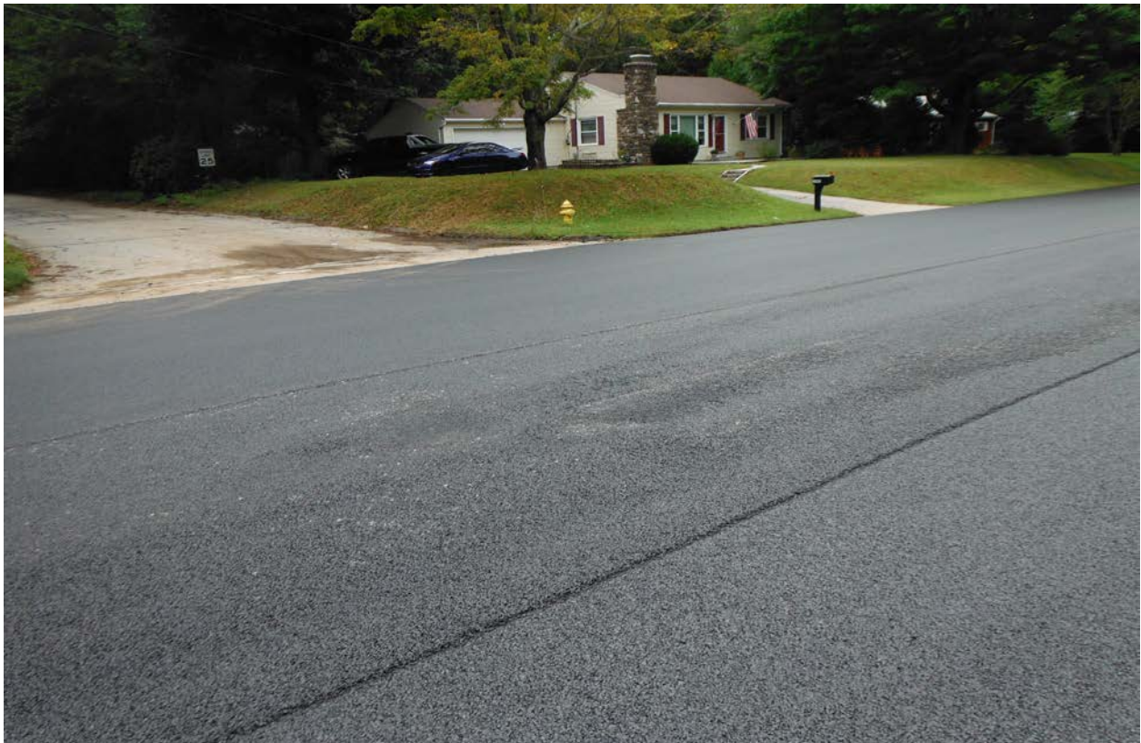
Figure 6. Surface Irregularities at Cardinal Lane Intersection
