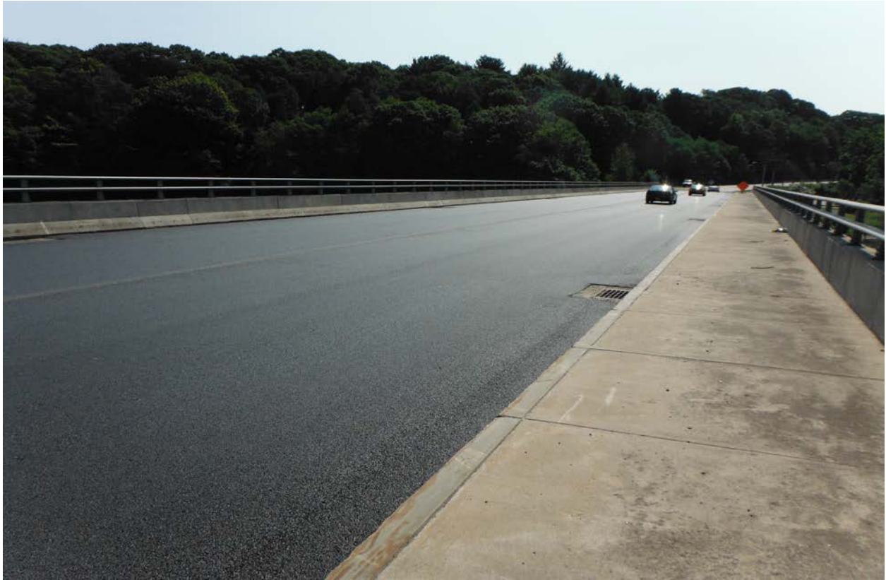
Figure 4. General Condition of the HFTL Mix
