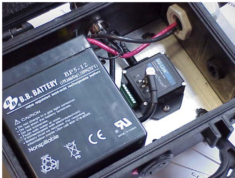
Figure 6. Typical Sensor Containment Box
