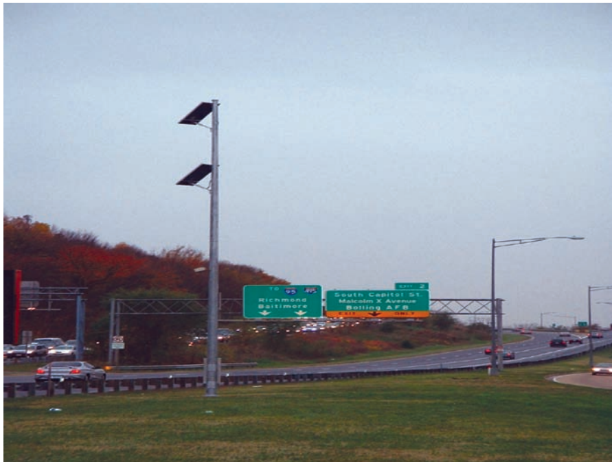
Figure 20: Typical Sensor Station Installation (MT, 2005)
