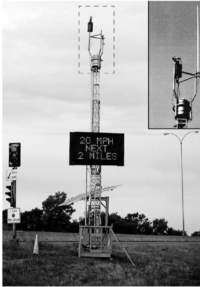
Figure 9: Smart Work Zone System Photo courtesy of SRF Consulting Group, Inc.
