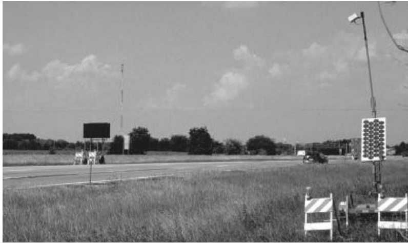
Figure 7: RTTCS Components - PVMS and Traffic Sensor with Solar Array Photo courtesy of FHWA (Federal Highway Administration)
