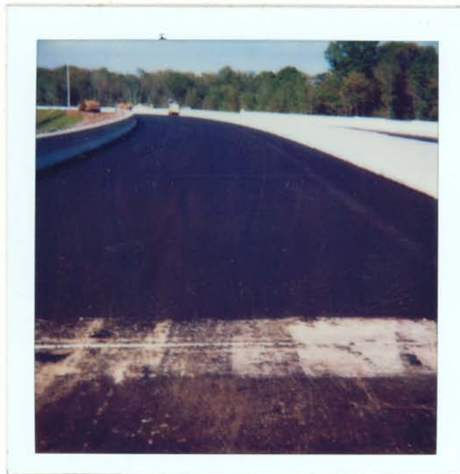
Fig. 4. View of deck on test side of bridge. Top course containing Verglimit has just been completed.
