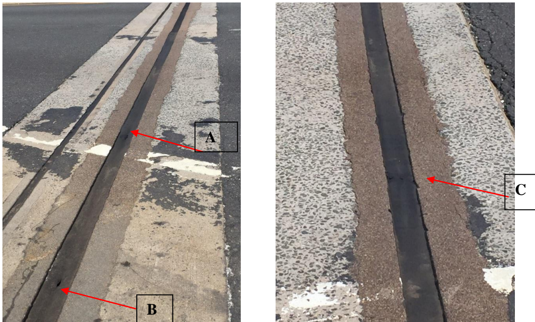
Figure 71: Visual observation of damage on Route 291 Bridge
