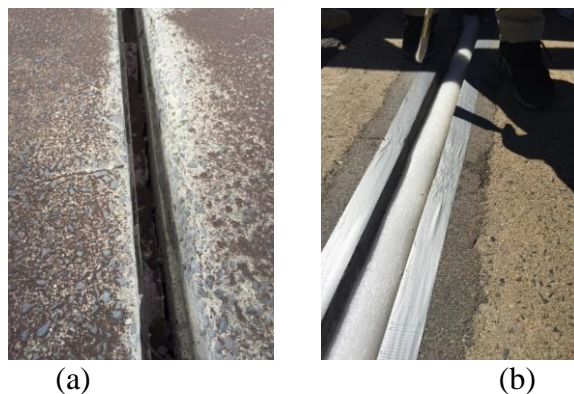
Figure 49: Overview of the joint on Route 6 Bridge (a) before backer rod installation and (b) after installation
