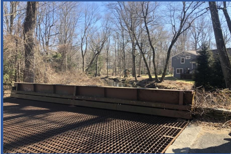
Open grid deck, southern through girder, rub rails, and timber guide rail bridge attachment.
