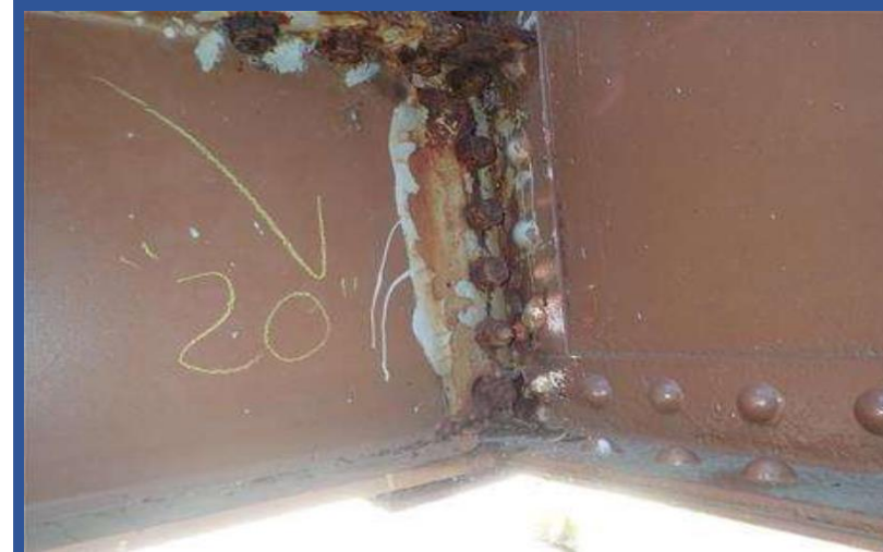
Superstructure Deterioration – Floorbeam / Girder connection
