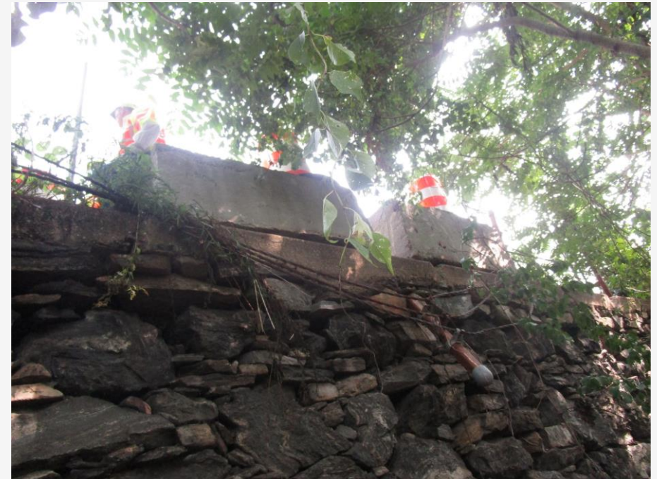
3 Cable rail and retaining wall damage from 2019 crash
