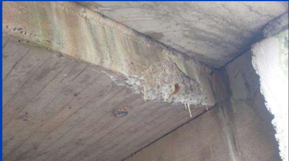
Scale on the underside of deck.
