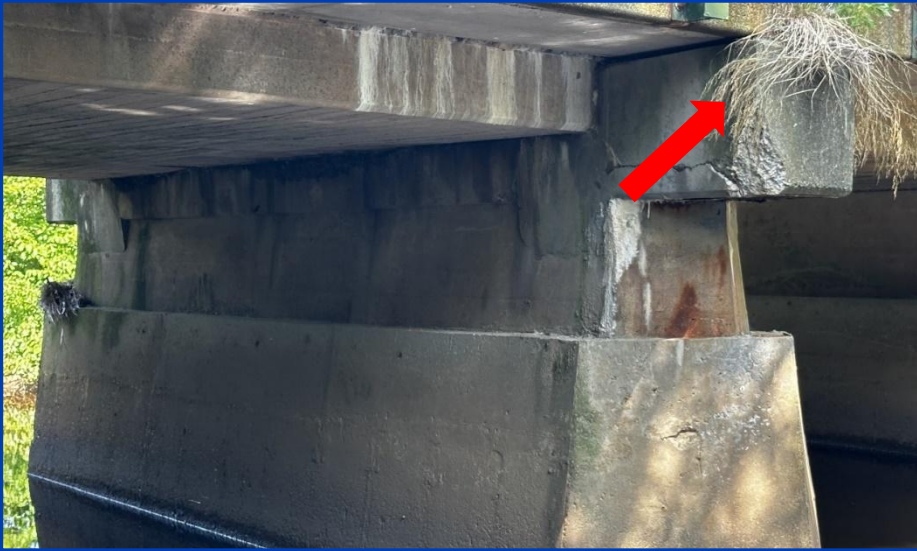
Center pier from downstream. Note: Spall on pier cap.
