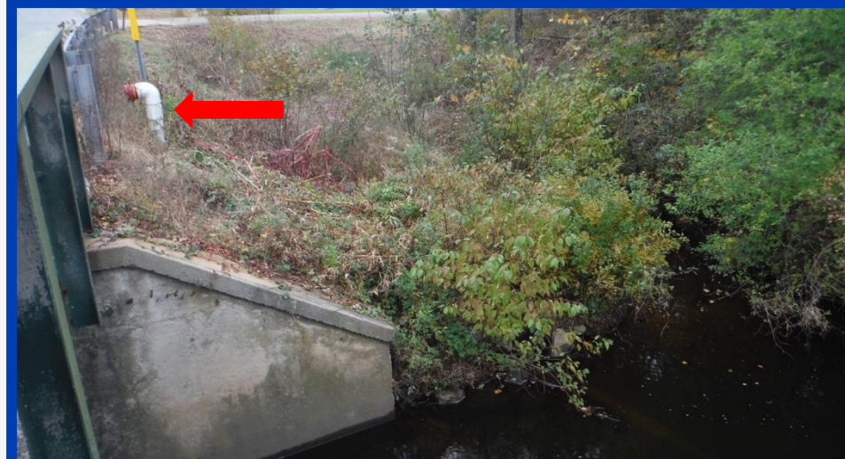
Dry hydrant located near the southeast wingwall.
