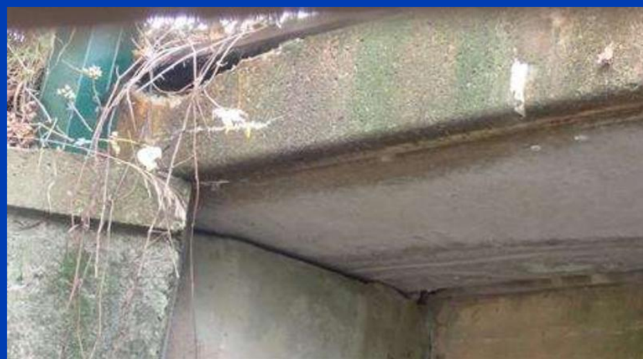
Spall in deck at northeast fascia of prestressed concrete deck unit.
