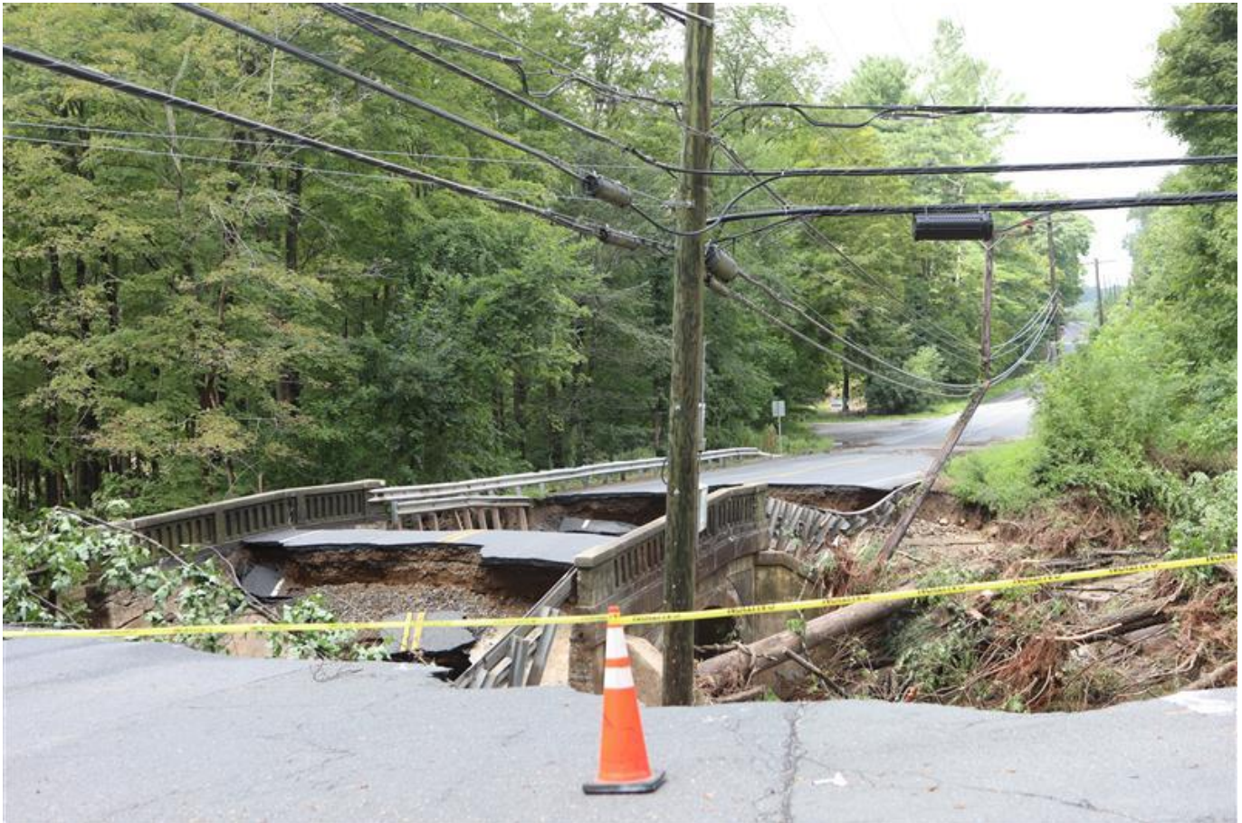
Figure 15: Washout in Oxford, CT. August 2024.
