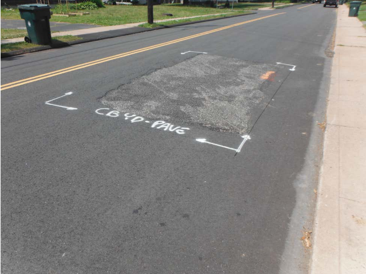
Figure 11. Lenox Street Water Main Break Patch Section
