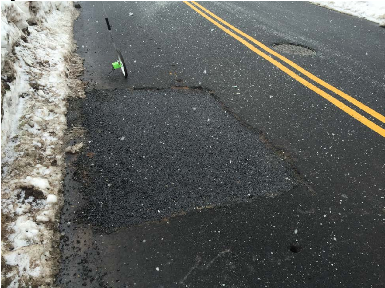
Figure 12. Lenox Street 2014 – 2015 Patched Section
