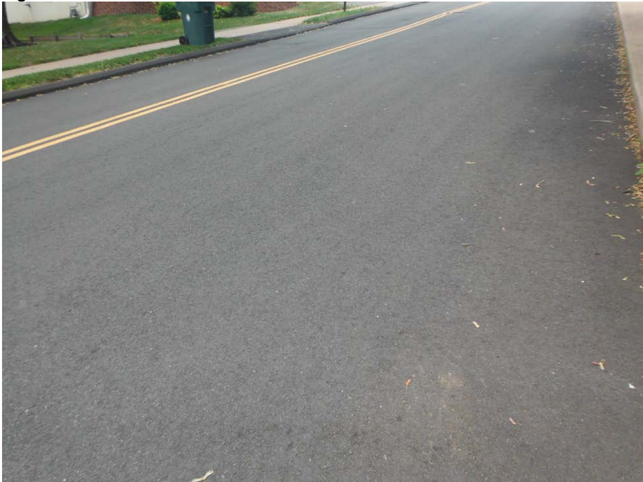
Figure 15. Lenox Street June 2014 General Surface Condition
