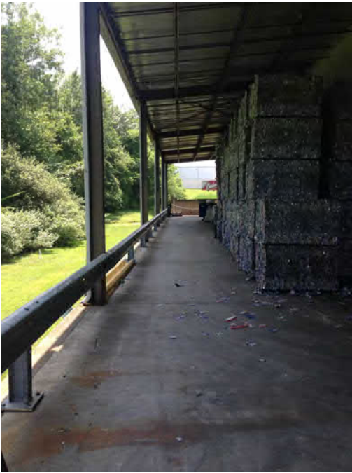
Photo 11: View along eastern side of building under covered storage area (facing southwest)
