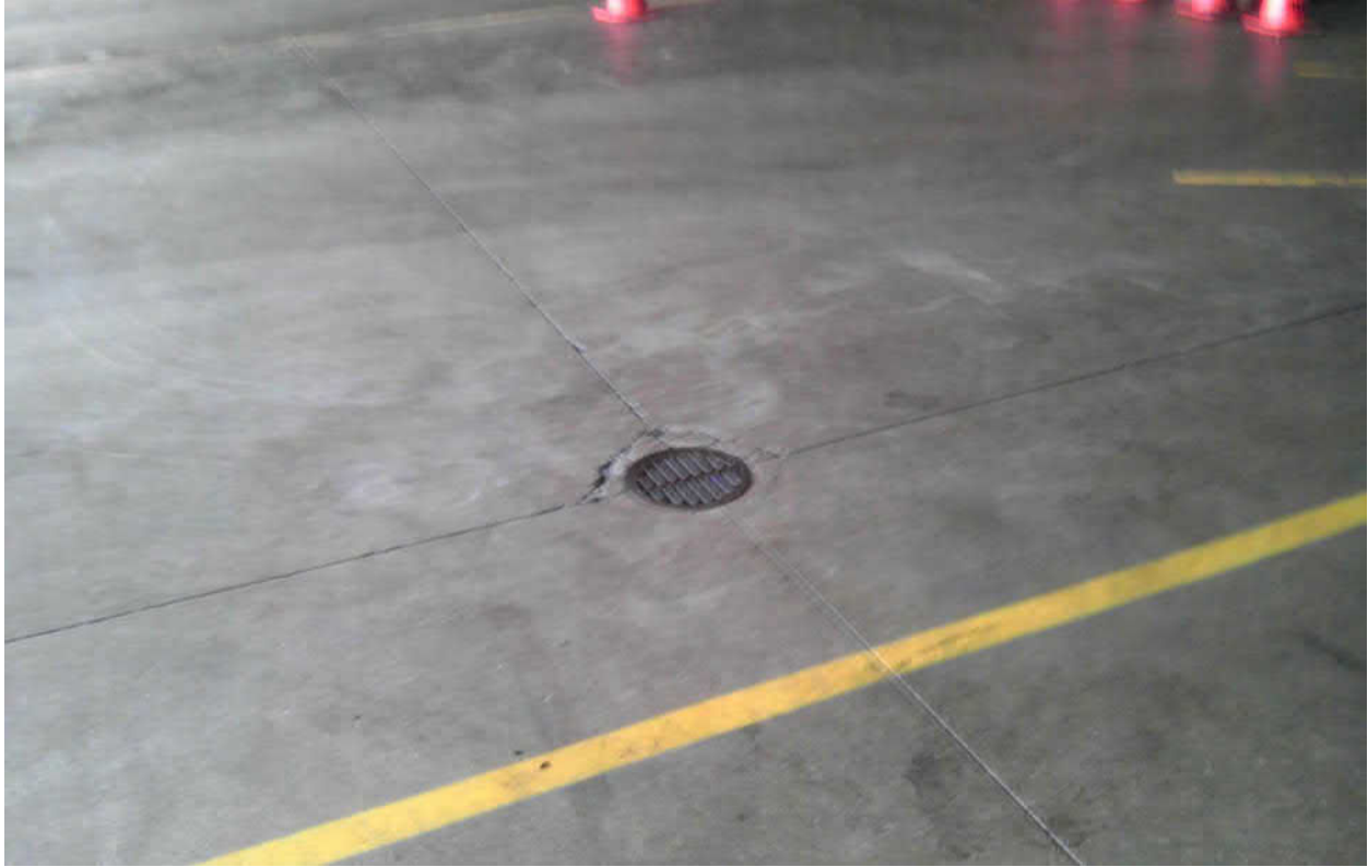
Typical floor drain inside can recycling center building
