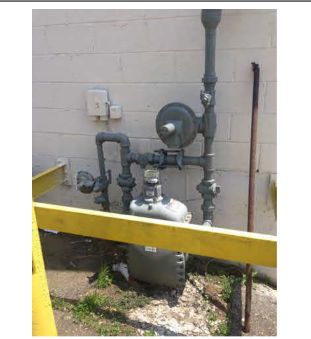
Photo 4: View of gas meter along western side of building (facing southeast)
