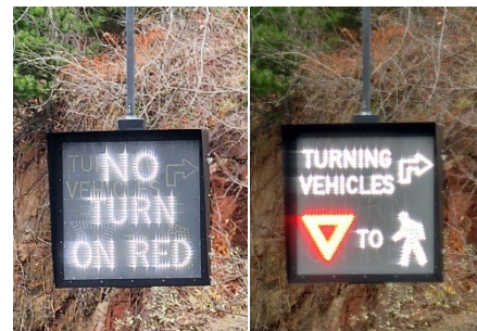
Figure 3: A Dynamic RTOR Message Sign in Manchester
