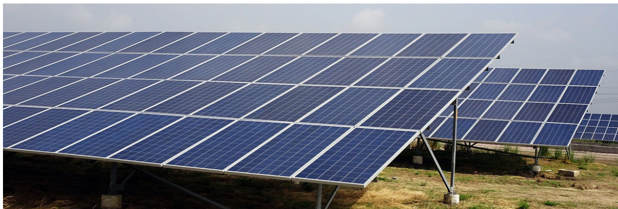
Figure 4.1: Solar installations will take advantage of potentially underutilized space.
