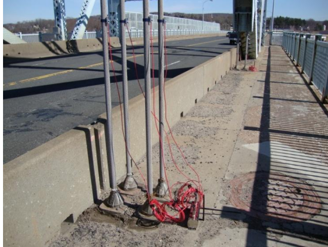
Figure 3. BDI STS-WiFi System Deployed on Arrigoni Bridge
