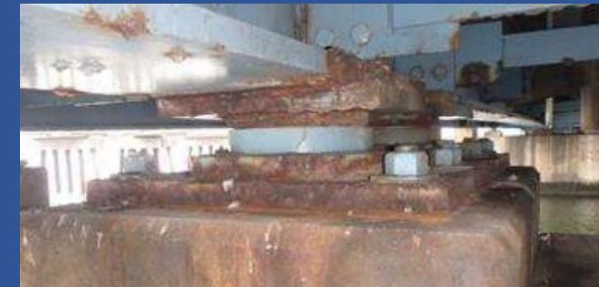
Rust at approach span bearing plate
