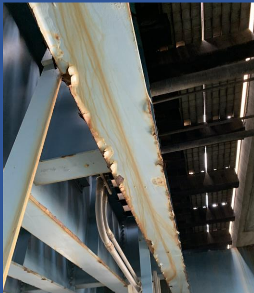
Peeling paint at railroad girder
