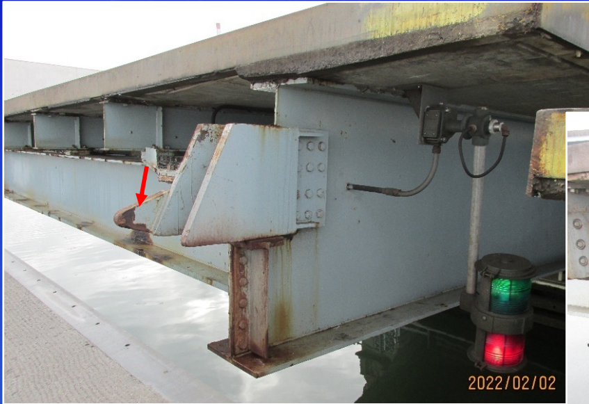
Jaw with added Extension Bar. Will be Replaced with New Lock Bar type Motor Actuated Span Locks
