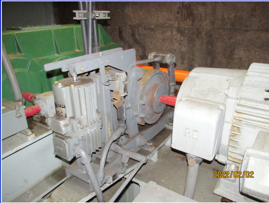
Primary Gear Reducer (green), Brake (center), Motor (right). Replace as new.
