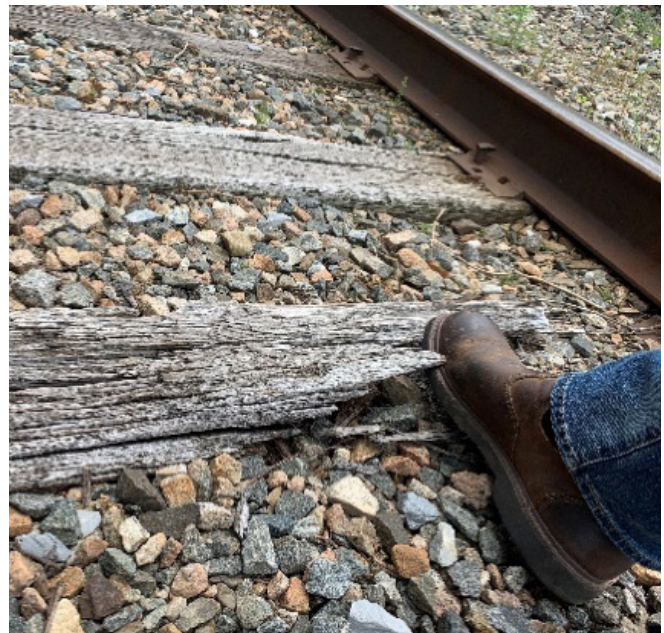
Figure 12 Wooden Ties with Severe Rotting
