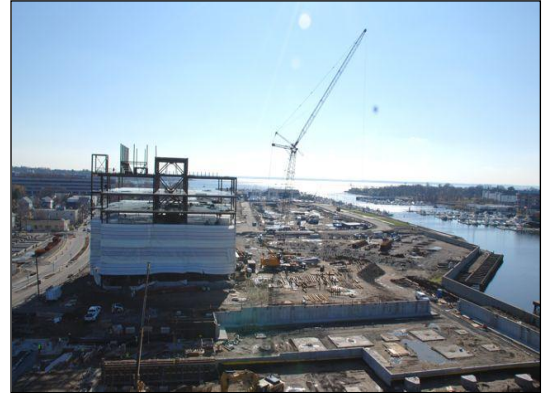
Overhead View of Construction at Harbor Point Photo Courtesy of: Harbor Point Development
