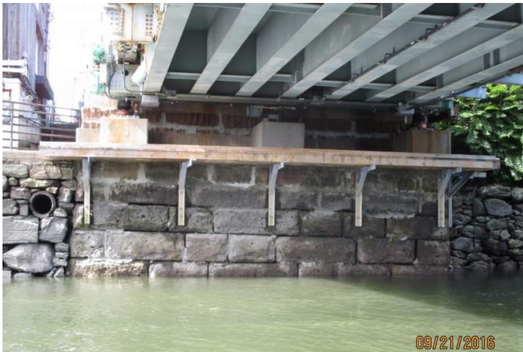
Image 9: Western abutment of Bridge #01349. The original ashlar masonry is visible. Reinforced concrete was introduced on top of the abutment in 1993 to raise the bridge clearance above the water and facilitate river traffic. The outriggers and catwalk allow access to the screw jacks that raise and lower the swing span when it is operated.
