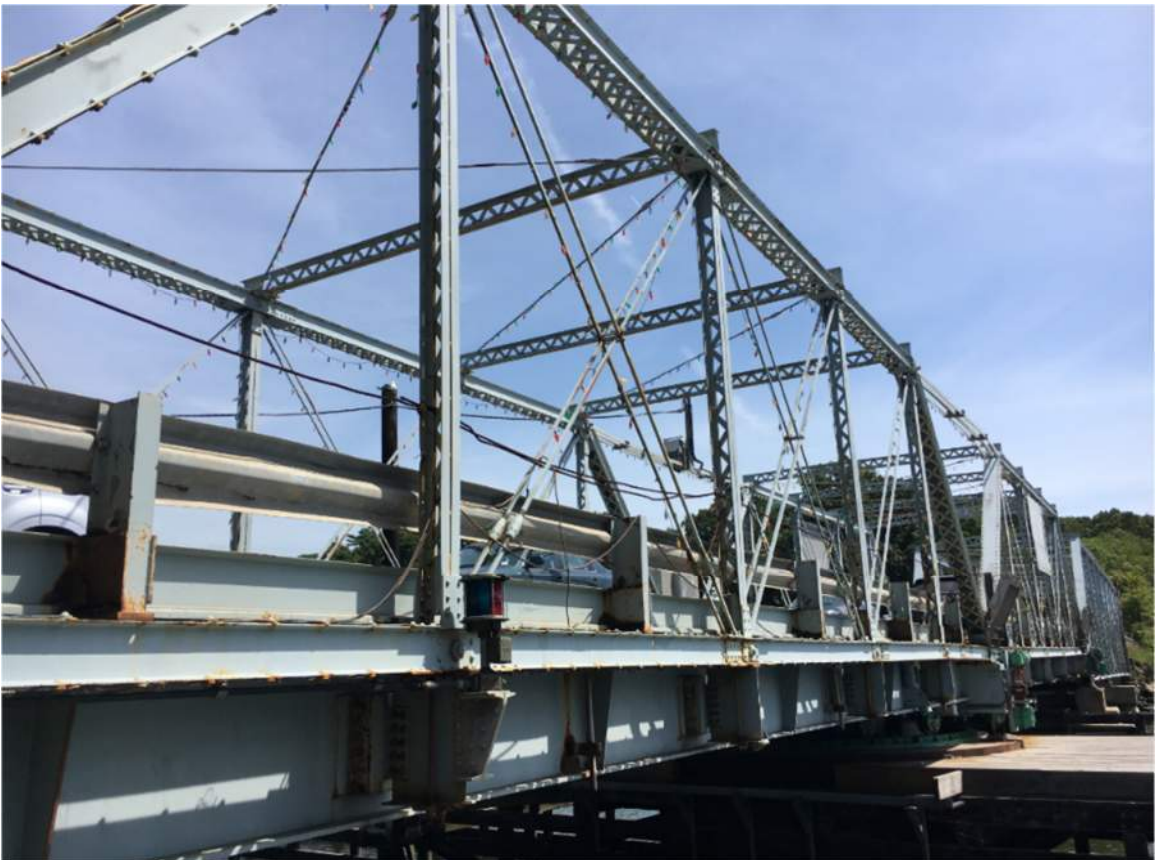
Image 2: Existing metal beam guiderail abutting the decorative trusses. When the guiderail is struck, the truss members restrict any deflection and the force of the impact is transferred to the truss.
