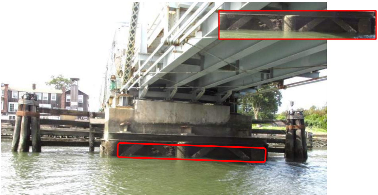
Image 11: Eastern face of Pier 2. The original masonry is outlined in red. It is obscured by modern pilings, a concrete cap and the timber cribbing that protects the western side of the pier. The detail in the upper right corner has been enhanced to highlight the masonry in the shadows.
