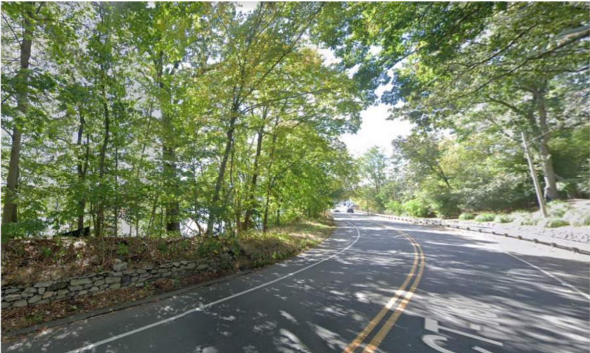
Image 6: Stone wall on southern side of Route 136. This wall abuts the property line of 12 Bridge Street. The wall terminates 375 feet east of Bridge #01349, which is located beyond the curve in Route 136.
