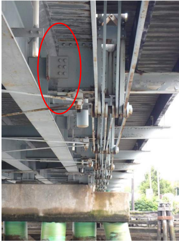
Image 6: The original beams of the truss were oriented perpendicular to the roadway. In 1991, they were cut and attached to the new superstructure beams (outlined in red), which are oriented parallel to the roadway.
