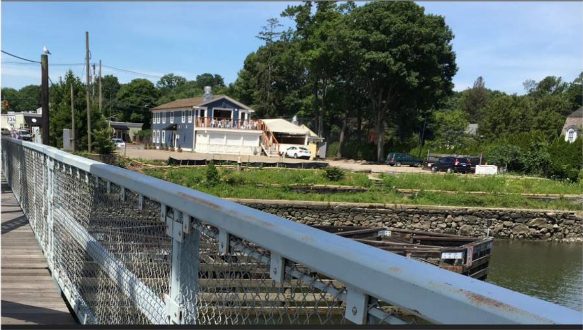
Image 9: Masonry retaining wall on the west bank of the Saugatuck River, viewed from Bridge #01349.
