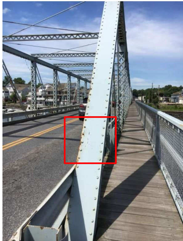
Image 13: There are a few locations where the original rivets have been replaced with bolts (see inset). However, almost all of the original rivets remain intact.
