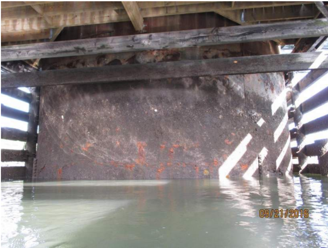
Image 10: Detail of pivot pier. In 1952, the original masonry pier was encased in a sheet metal form which was filled with concrete.
