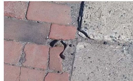
Figure 8. Sign Stub Trip Hazard
