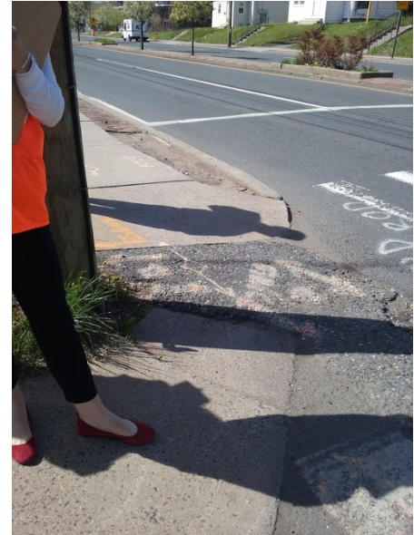
Figure 7. Narrow Sidewalk Ramp with Inadequate Landing
