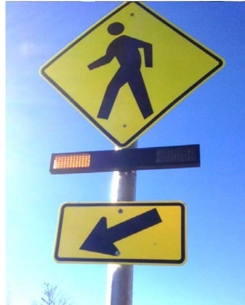
Figure 23. Typical Flashing Beacon
