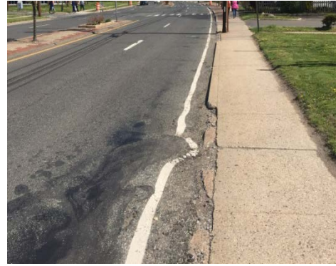
Figure 16. Damaged Curb and Sidewalk
