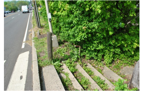
Figure 12 Sidewalk constrained by slope
