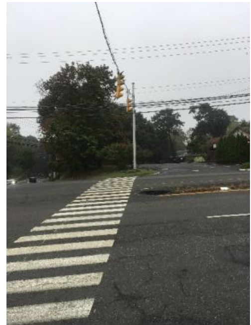
Figure 11. Crosswalk Missing ADA Ramp
