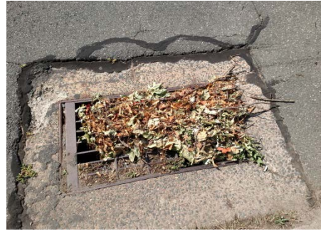
Figure 9. Clogged Non-Bicycle Friendly Catch Basin
