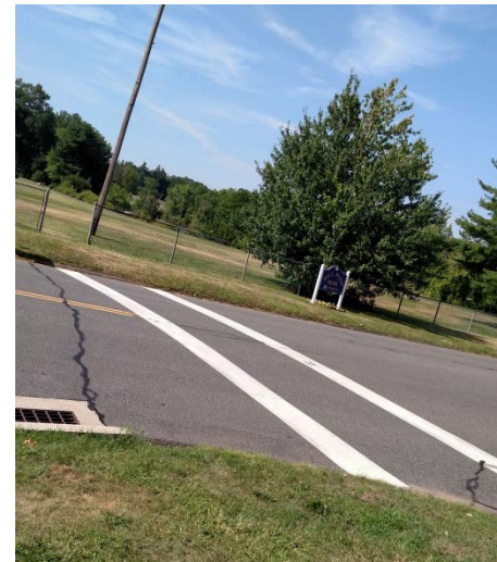
Figure 8. Crosswalk Ends in Grass
