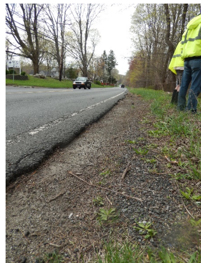
Figure 8: Pavement conditions along Route 37
