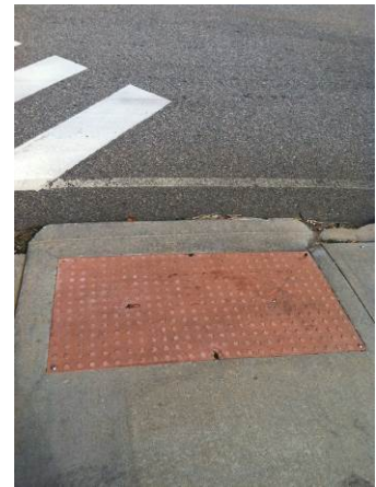
Figure 8. Worn Detectable Warning Strip
