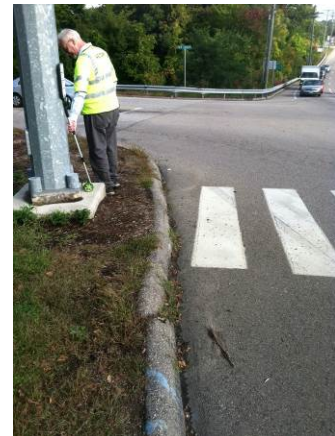
Figure 19. Guiderail Abutting Roadway; Lack of Ramp at Crosswalk
