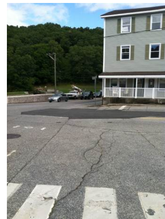
Figure 15. Broken Loop Detectors
