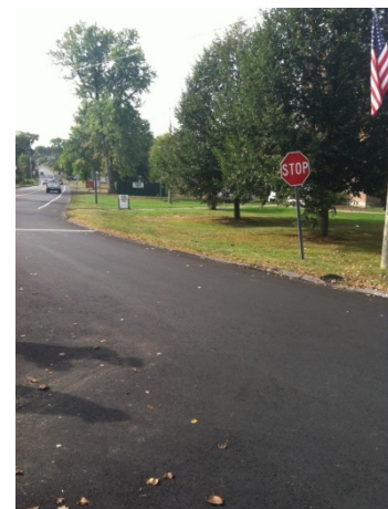
Figure 6. Stop Sign and Stop Bar not Aligned
