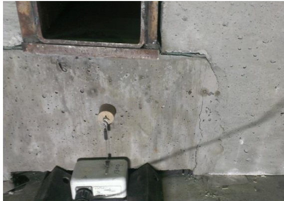
a) Propagation of crack
