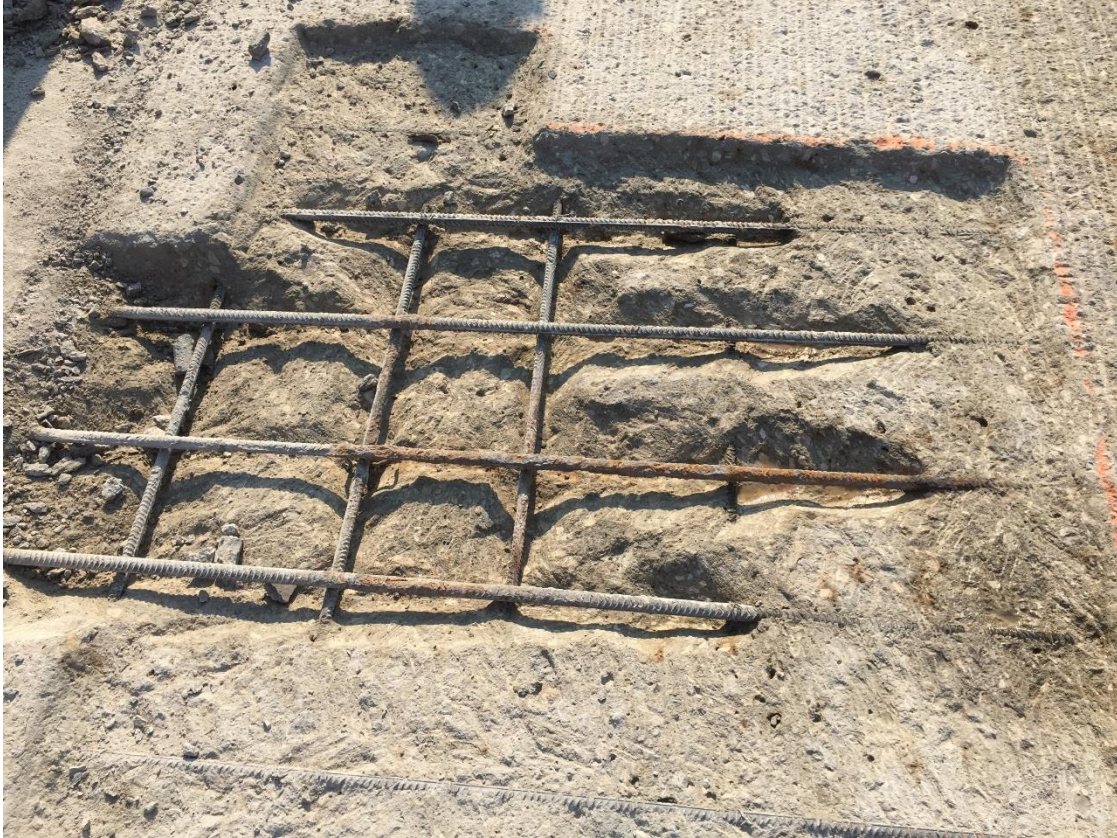
Figure 5. Deteriorated area of the deck after removal of the substrate concrete
