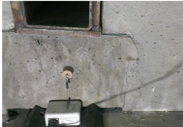
a) Propagation of crack
