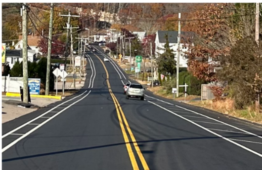
Figure 4: Buffered Outside Shoulder , Montville, CT - Image Credit: CTDOT Project Planning Unit. Buffered or "Visually Separated" Shoulder: Buffered or "Visually Separated" Shoulders can be an acceptable treatment for both cyclists and pedestrians in rural and suburban contexts without significant non-motorized generators. These facilities can be used on higher speed and/or volume rural roads where sidewalks and dedicated bicycle facilities are not present or warranted. The Buffer area should consist of two parallel white lines, 2' or more apart, and may include hatching in the buffer area.
