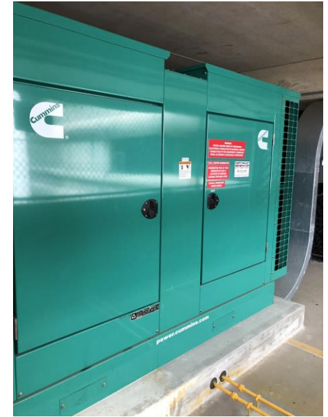
Generator Upgrade Stamford Government Center
