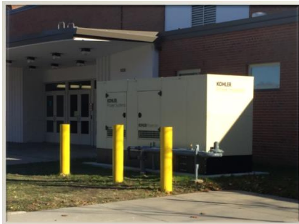
Essential Generator Jonathan Law High School, Milford
