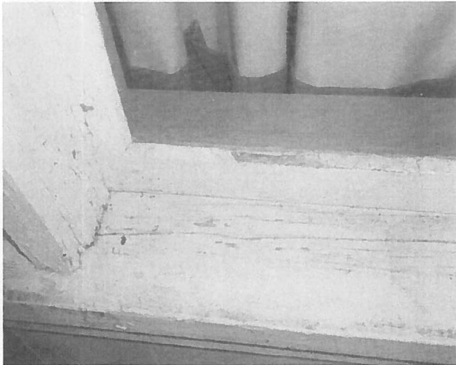
Defective Lead-Based Paint on Window Sill
