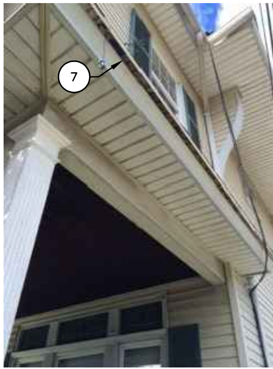
PHOTO 7 NON-INTACT LEADED SURFACE FRONT PORCH ROOF TRIM (N.T.S.)
