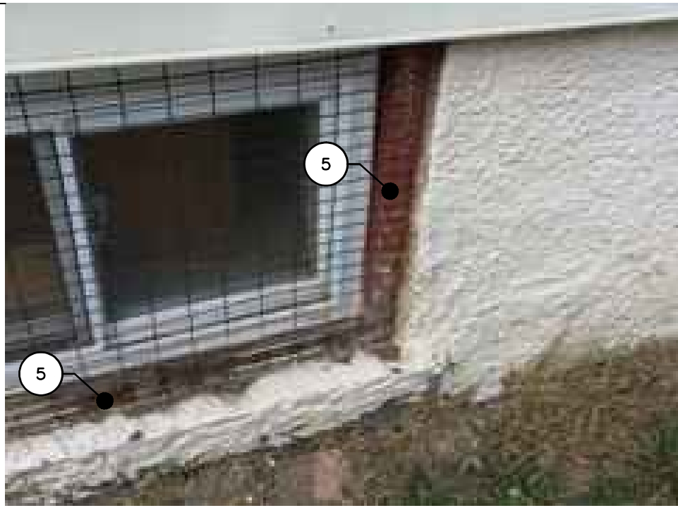
PHOTO 5 NON-INTACT LEADED SURFACE BASEMENT WINDOW TRIM ONE OF MULTIPLE WINDOWS SHOWN (N.T.S.)
