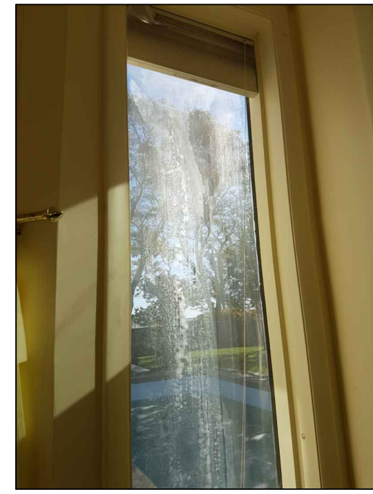
REPLACE INSULATING GLAZING UNIT IN BEDROOM 101 (INTERIOR VIEW) [ref. Keynote 2]
