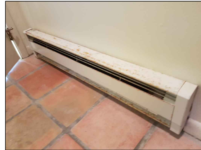
EXAMPLE OF TWO (2) BASEBOARD HEATERS TO BE REPLACED [ref. Keynote 4]
