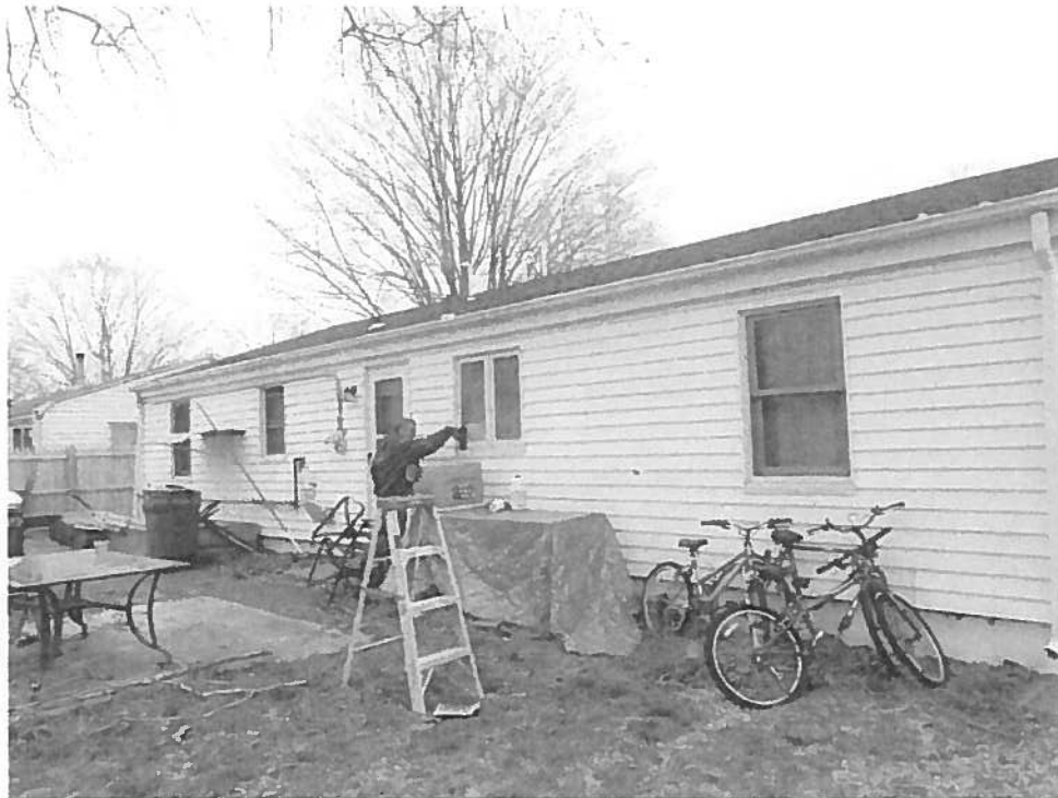
Side C Exterior (lead paint identified on upper face board)
