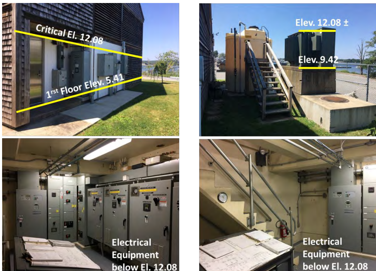
Figure 22 - Photos of Mago Point Wastewater Pump Station
