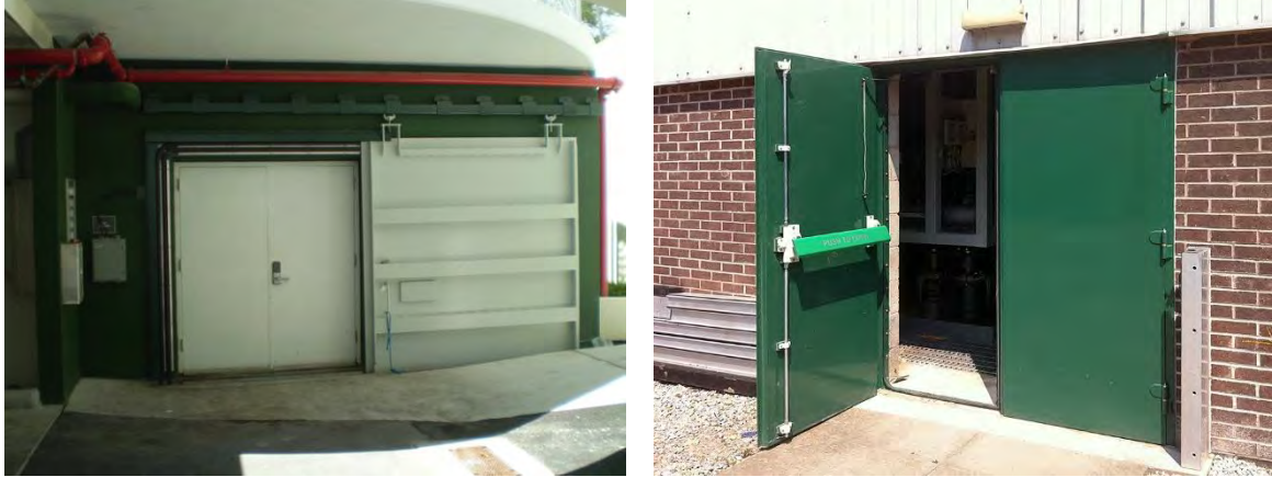
Figure 24 - Example of Sliding Flood Door (left) and Floodproof Double-Door (right)
