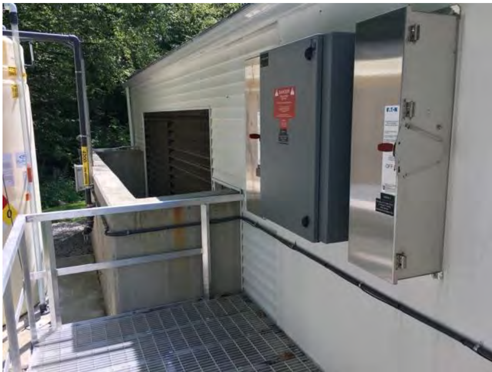
Figure 20 - Concrete Flood Wall and Raised Electrical Panels at Bolles Court Pump Station
