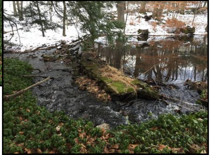
Photo No. 51 (Full dam span above, eroded portion right)
