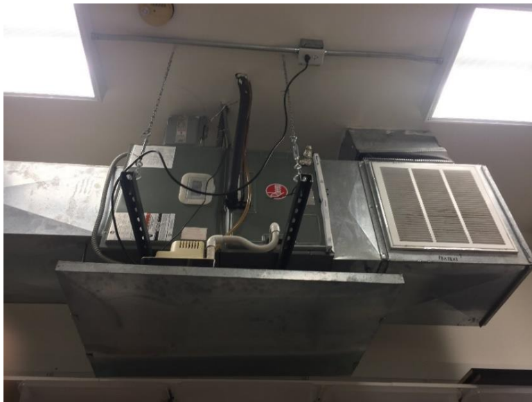
Image of elevated HVAC system on the first floor of building on Main St.
