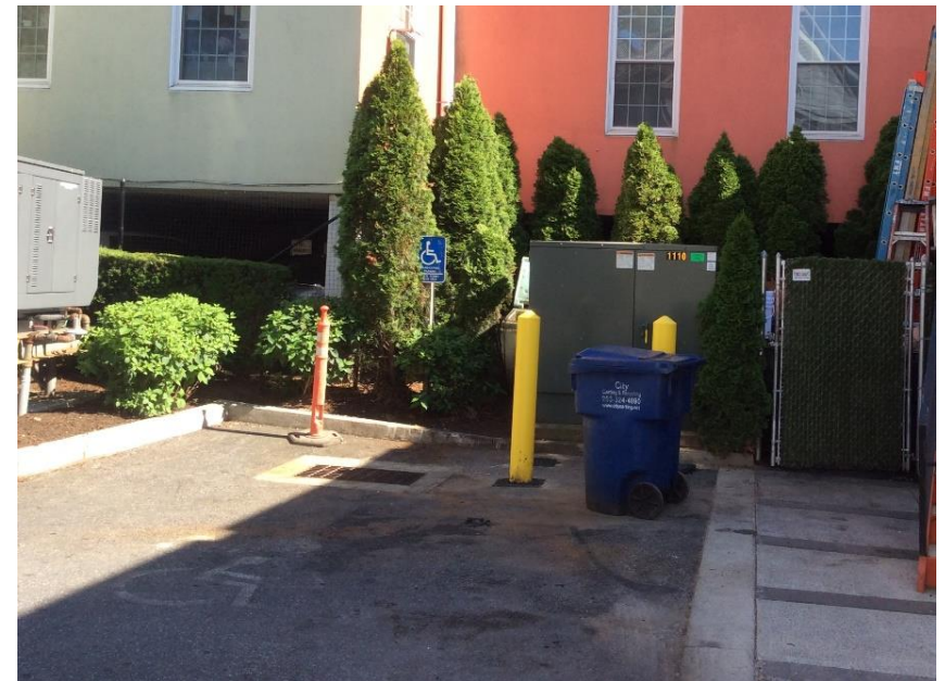
Image of Electrical Transformer near a catch basin in the back of 101 Post Road East
