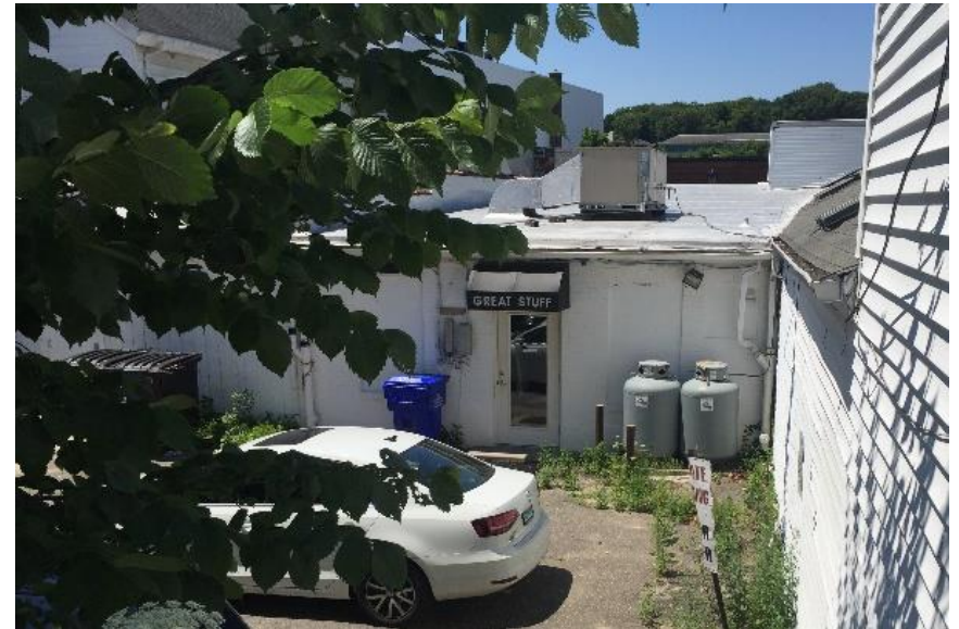
Image of HVAC system on the roof and propane tanks at grade behind Main St.
