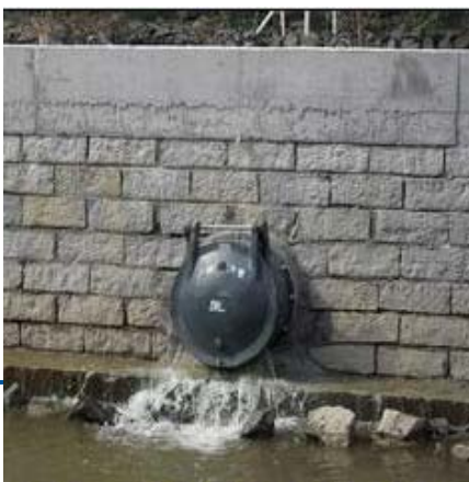
Stormwater Flap Gate
